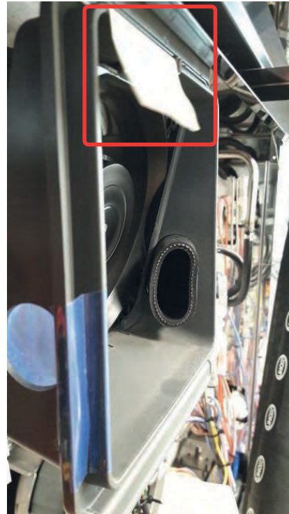
Test 2 Fan is running in the right direction
